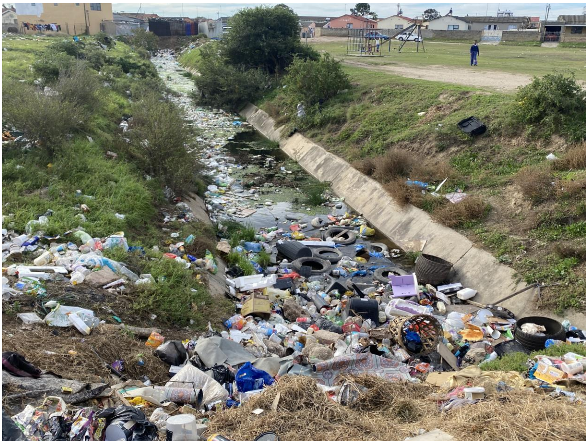
Figure 5.1. Pollution in the Swartkops canal running through Motherwell Township. © Sipesihle Booii
