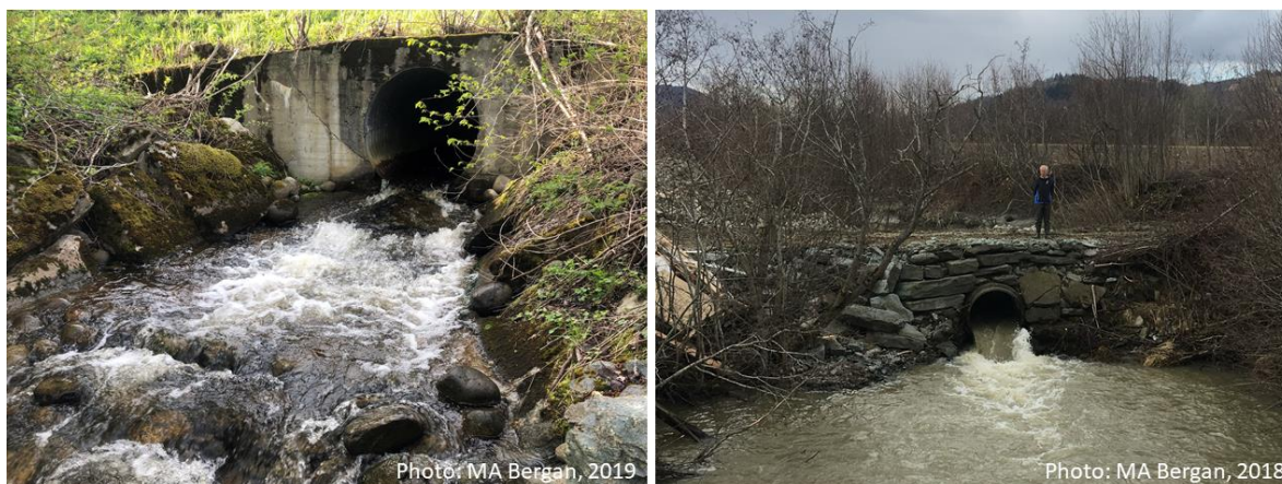
Figure 1. Examples of culverts: an old culvert under Fv 707 Leinstrandvegen over the Lauglobekken stream (left panel), and a culvert under a private road over the Eggbekken stream (right panel). All hotspots for spawning in both streams are located upstream of these culverts. In the case of Eggbekken, all sea trout spawning may collapse in some years due to this migration hindrance.
