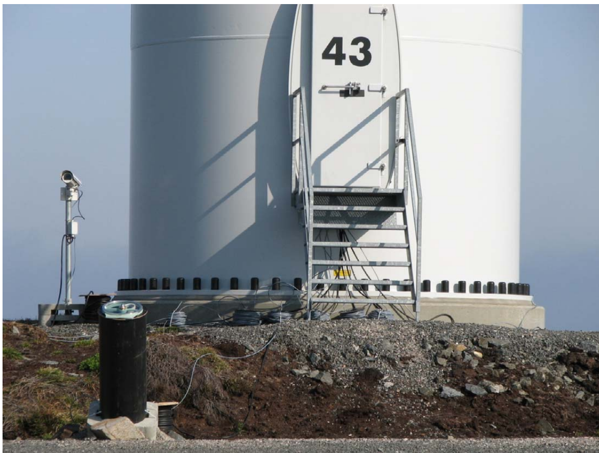
Figure 30. Camera system installed in connection to wind turbine 43. Photo: Kjetil Bevanger.
