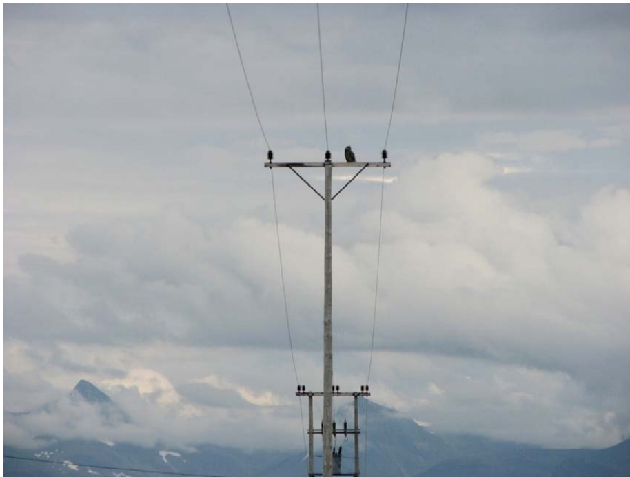
Figure 9. Eagle owl perching on the crossarm of a 22kV pole (no 148). Pole no 149 with pole mounted transformer in the background where bones of one dead eagle owl was found in July 2008. Two dead eagle owls were recorded beneath the same pole in spring 2005. Photo: Jan Ove Gjershaug.
