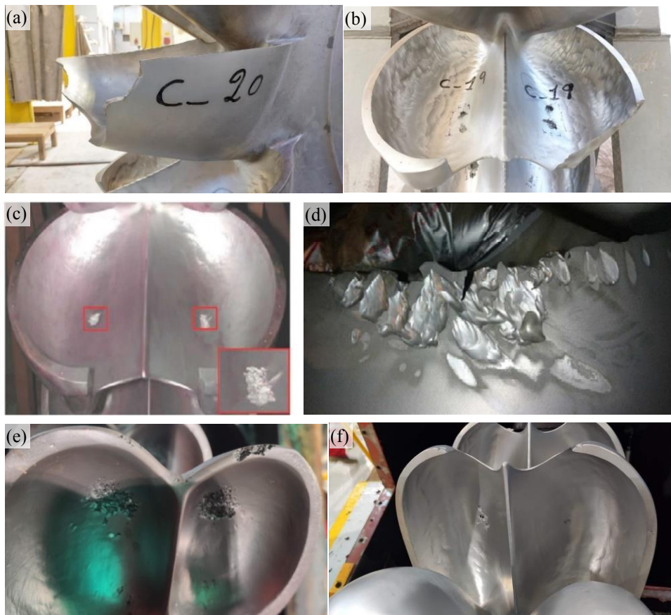
Figure 2. Cavitation on Pelton turbines. a & b) Cavitation on the inner surface of the bucket and break of a side of the outlet edge at Ancash-Peru. c) Cavitation on the inner surface, Smith [15]. d) Cavitation in the bucket splitter at Lima-Peru. e) Cavitation on the inner surface and lips of the bucket at Pasco-Peru. f) Cavitation on the inner surface of the bucket at Pasco-Peru.
