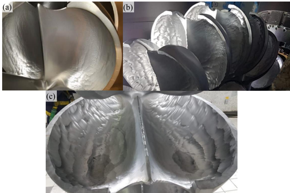
Figure 3. Regular erosion with starting of cavitation in Pelton turbine buckets. a) Runner after one year of operation at Pasco, Peru. b & c) Runner after four months of the rainy season at Ancash, Peru.
