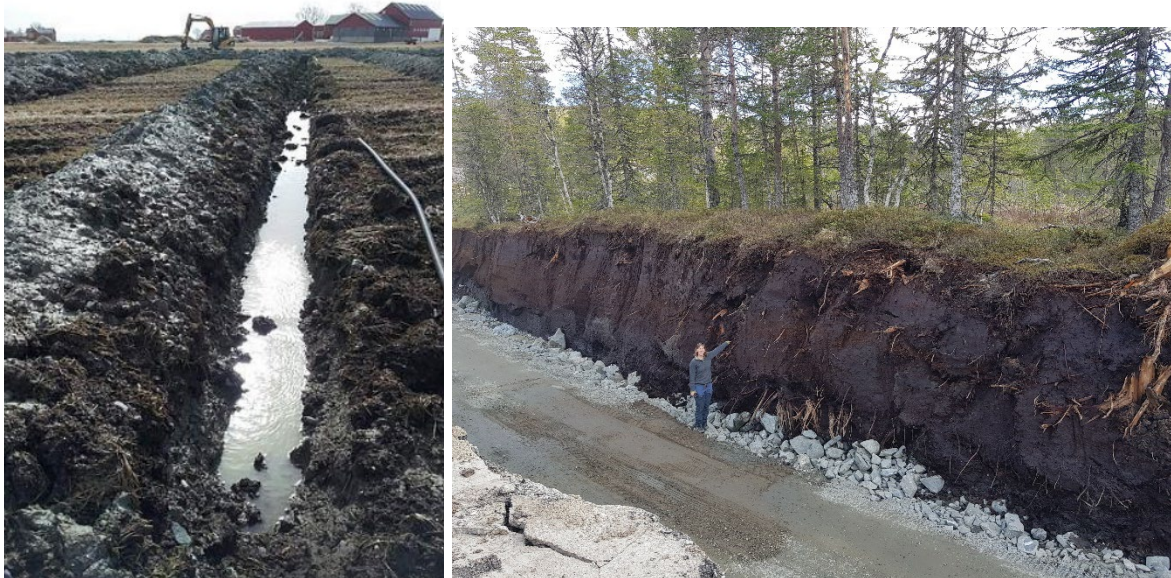
Figure 1. a) Agricultural peatland drained with ditch. b) Excavation of peatland for an access road. © Magni Olsen Kyrkjeide
