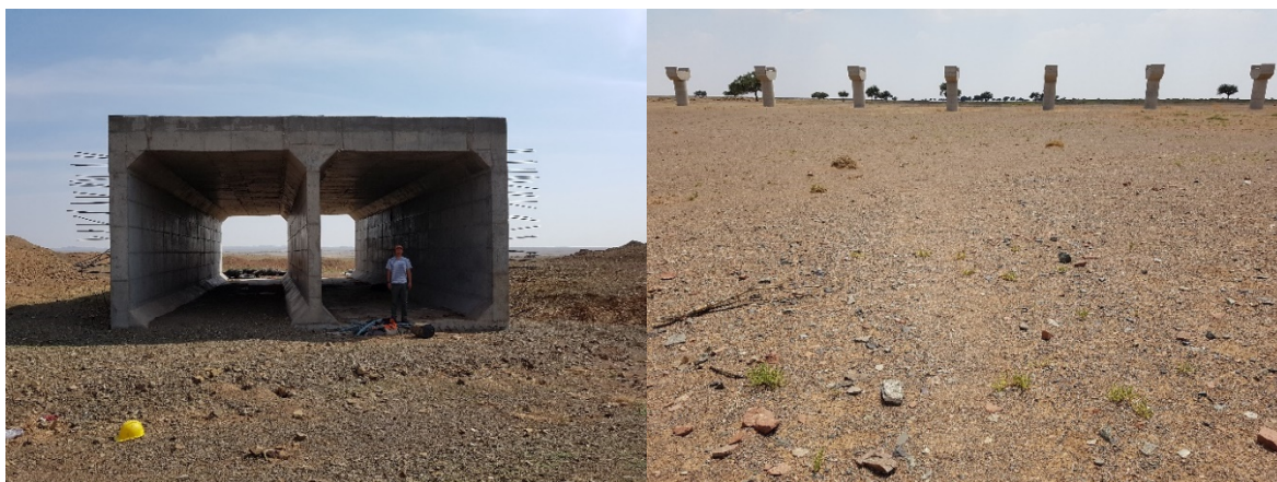
Figure 15: Crossing crossings structures to be implemented along the Tavan Tolgai - Gashuun Sukhait railway corridor (status: July 2017). Whether these crossings will also work for khulan and other wildlife is unknown. Note: the dimensions of the box culverts do not comply with the Mongolian standards for wildlife crossings which require a minimum height of 3m and a minimum undissected width of 10m. Photo: P. Kaczensky
