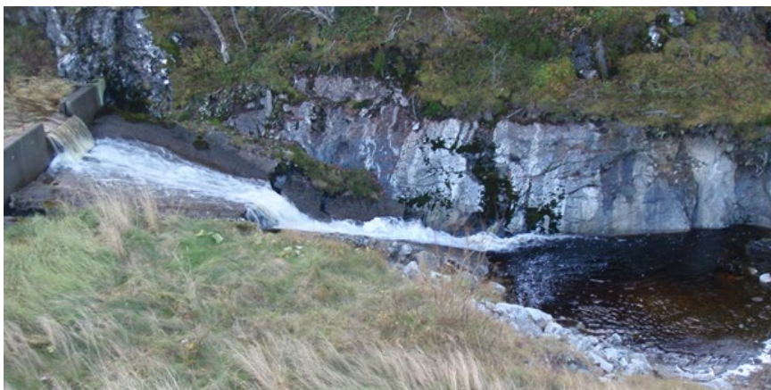
Figure 8. A concrete dam with a downstream chute at the outlet of Dragvatnet. Photo: © Morten Andre Bergan.
