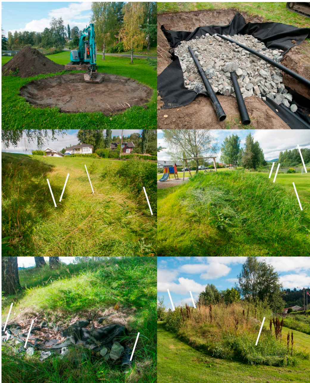
Figure A2. Photos of excavator at work during construction of Hotel 2 ( top left ), drainage pipes, geotextiles and rocks of Hotel 1 ( top right ), and final result of Hotel 1 ( mid left ), Hotel 2 ( mid right ), Hotel 3 ( bottom left ) and Hotel 4 ( bottom right ).
