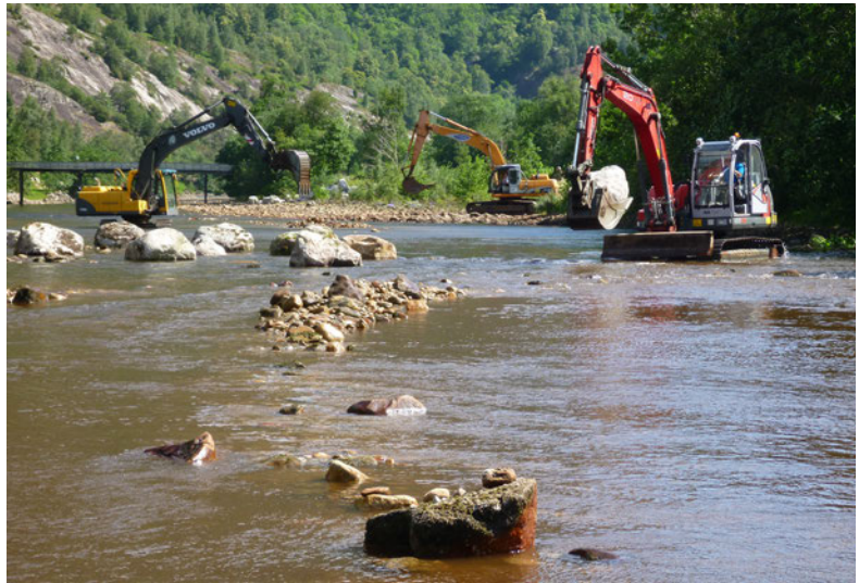
Figure 17. An example of gravel laying designed to create shelter and a more varied hydraulic environment along a uniform and channelled reach. From Frafjordelva river in Rogaland county, Norway. Photo: Ulrich Pulg
