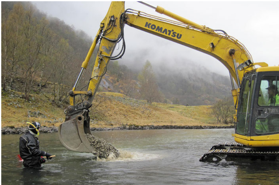
Figure 16. Installing spawning gravel using an excavator (from the Aurlandselva river in Norway). Trained personnel in snorkelling gear guide the operator as to volume and location, and then spread the gravel using scrapers and rakes. Photo: Bjørn Barlaup
